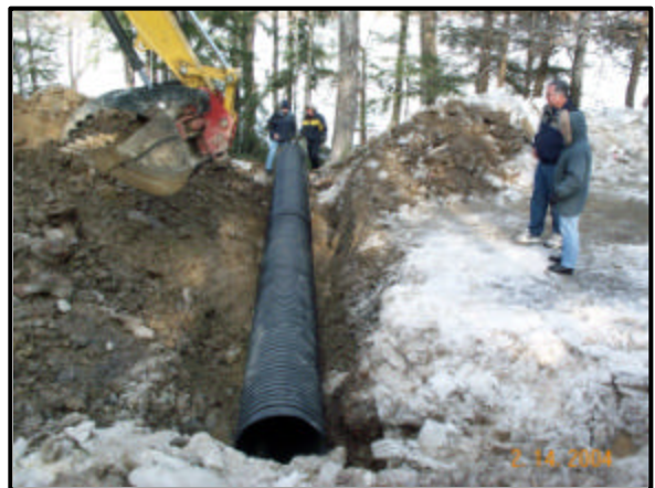
Sheldon Beal, Dave Brooks, Bob Beal and Edith Brooks observed the placement of the culvert in the trench near the Ellis camp.
